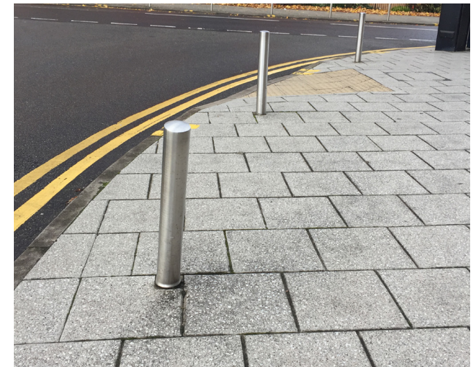
Existing slender stainless steel bollards. When the use of bollard cannot be avoided, similar bollards to these ones could be used.
